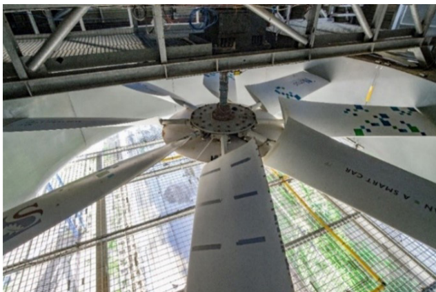
Fig. 3 Photo of the installed 24 ft M-fan
