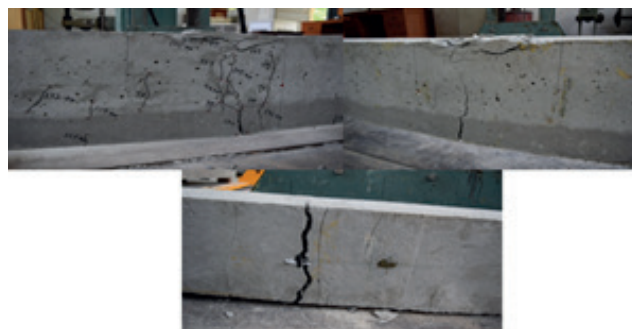
Fig. 14 Cracks formation and their distribution in RECC 75 beam
