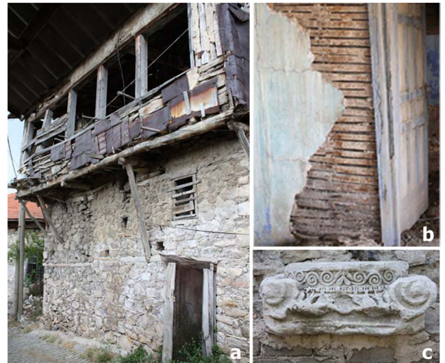
Fig. 7 (a) Housing unit with hybrid construction technique, (b) timber frame and timber lath construction system, (c) reused materials on the exterior wall of the housing
