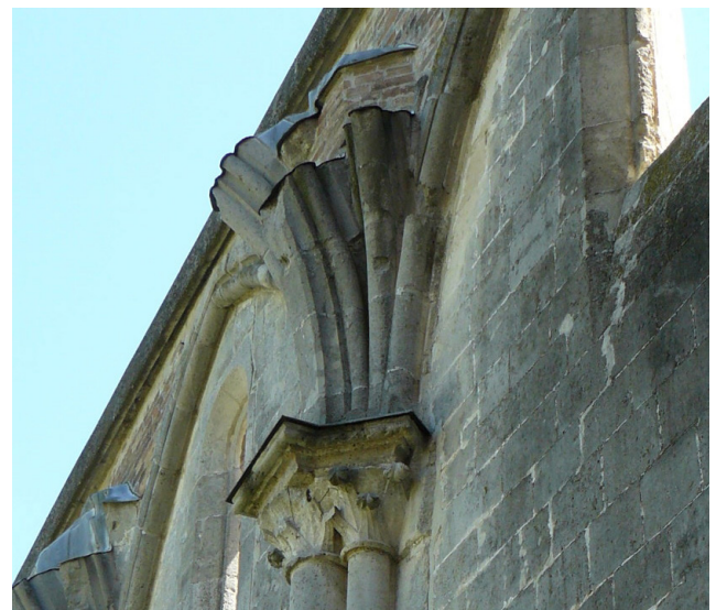
Fig. 13 Tas-de-charge type vault springer in the nave of the Church of Zsámbék.
