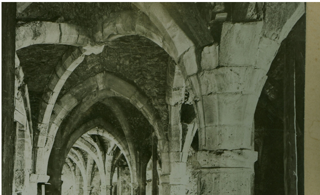
Fig. 14 Tas-de-charge type vault springers in the knight hall of the Castle of Léka (Plan Collection and Archives of BME Department of History of Architecture and Monument Preservation, ref. no. 800828).
